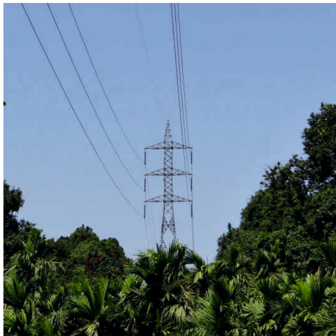
Energy Transmission Line Saltinho – Bambadinca | 110 kV | Guinea - Bissau Client: UNPD Tender Design: 1992/1994
