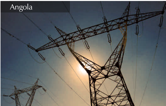
High Voltage Energy Transmission Line, at 220 kV, between Dundo and Luena - Empresa Nacional de Electricidade – E.P. | Angola | 2013
